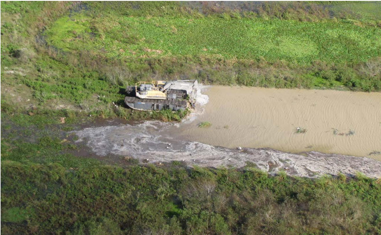
Aerial view of STA-1E Cell 6 refurbishments. Photo illustrates degrade of remnant farm berms using an amphibious excavator that digs up the berm material and drops it into the adjacent ditch as it advances backward (to the left).
