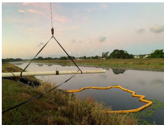
Figure 11. Discharge pipe set-up to discharge into the canal with silt fence in
