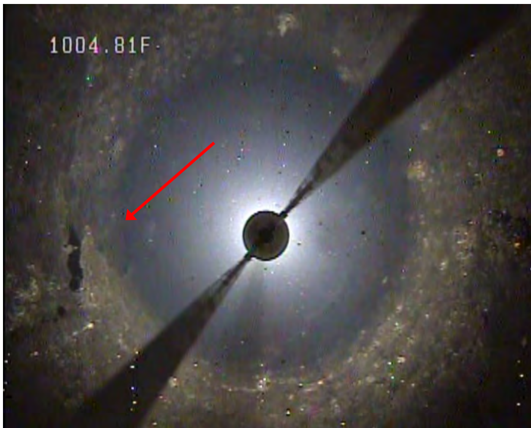
Figure 4. Spalling and peeling from casing wall at 1,005 ft bpl.
