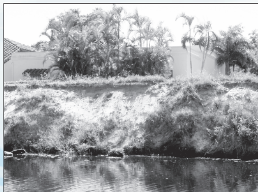
The Canal Bank Stabilization project will repair banks along the Hillsboro Canal and dredge a 1.3-mile section — from about Military Trail to Powerline Road — to ensure water can be moved through the canal to maximize flood protection.
