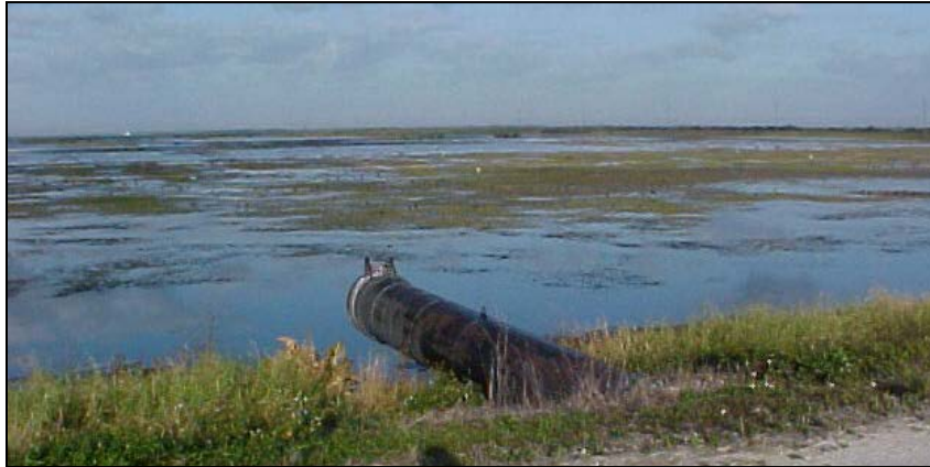
Figure 3. Pump Station Outlet
