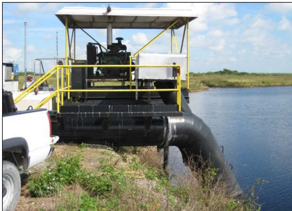
Figure 2. Pump Station Inlet
