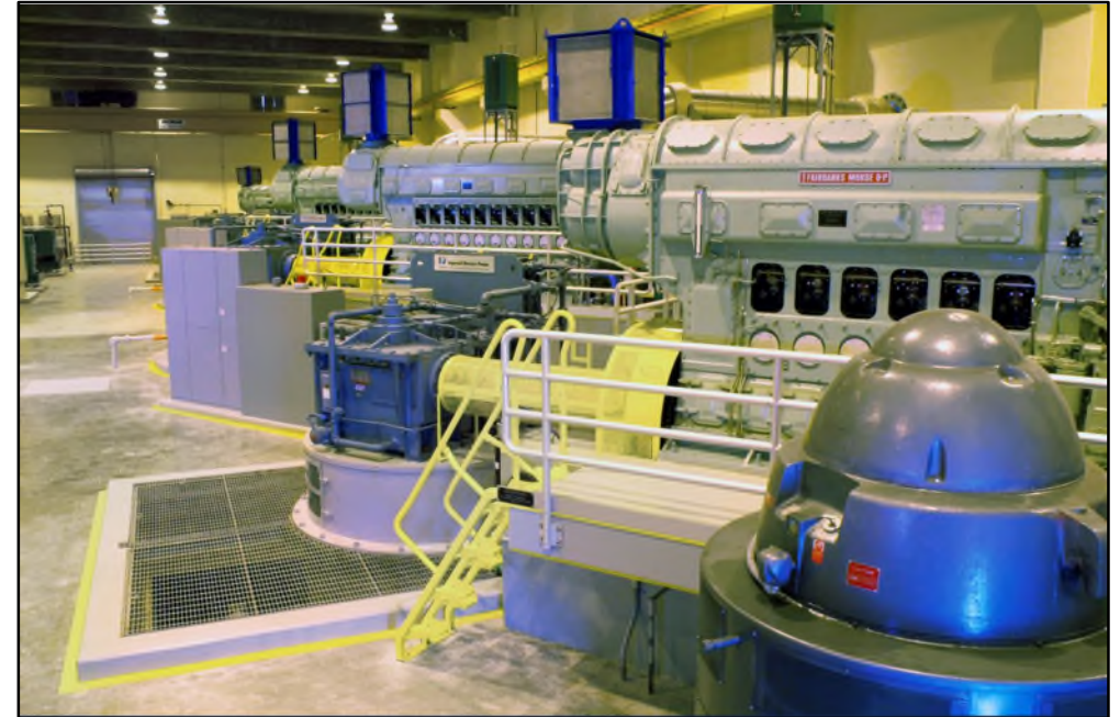
SFWMD Pump Stations provide important flood protection to many South Florida communities.
