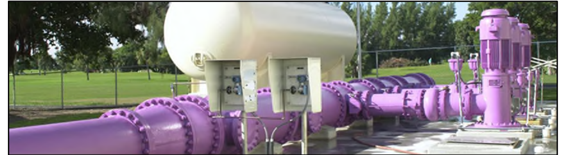
Reclaimed Water is often recognized by the use of purple pipes
